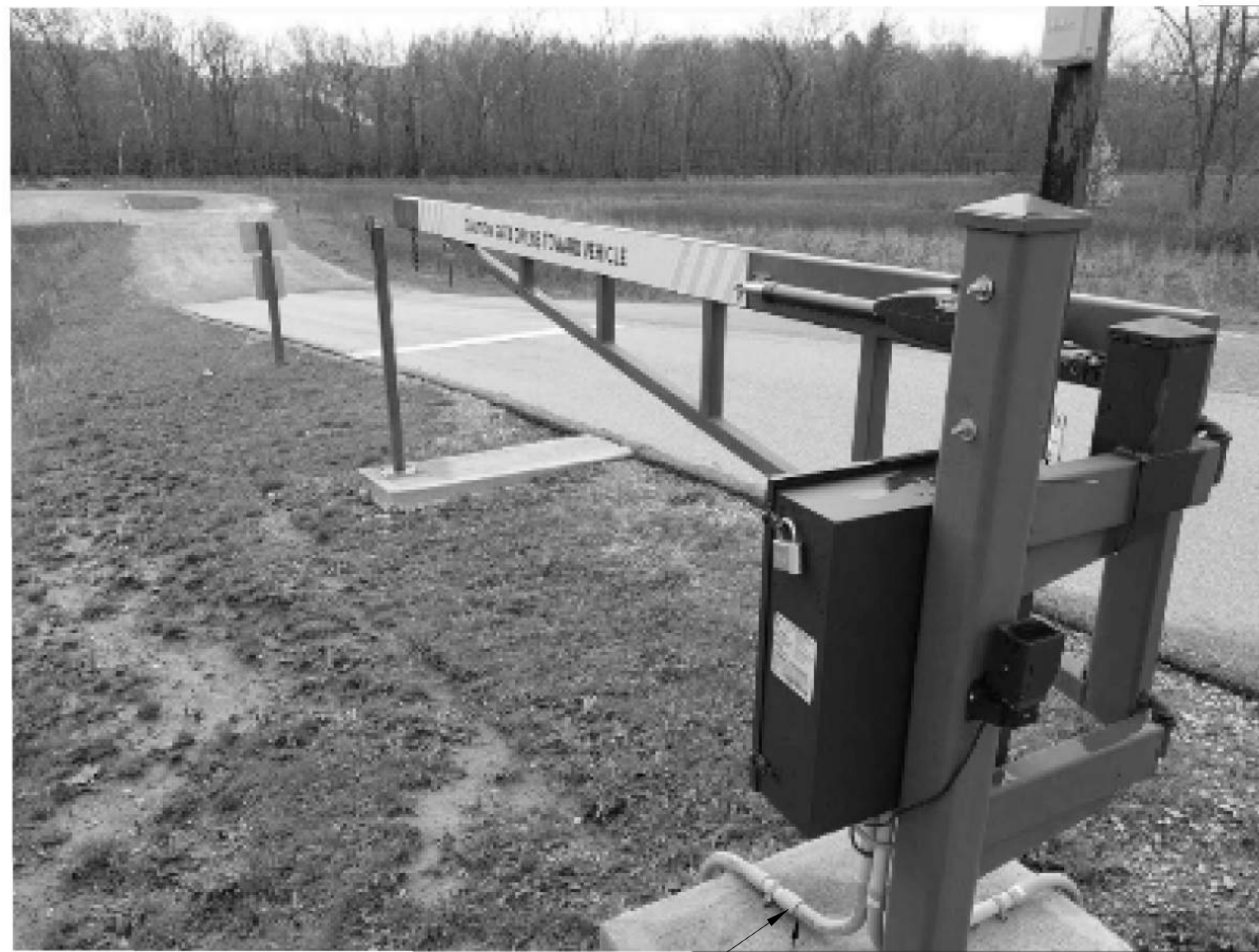
CONDUIT TO AUTOMATIC GATE OPENER EXIT SENSOR
